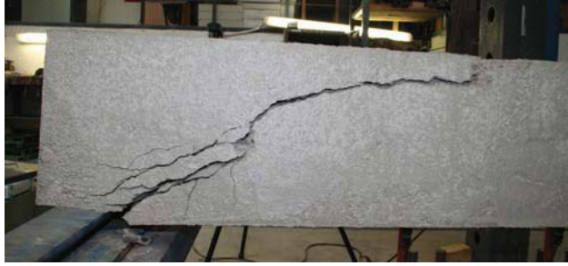
Figure 6. Cracked beam with GFRP shear reinforcement
