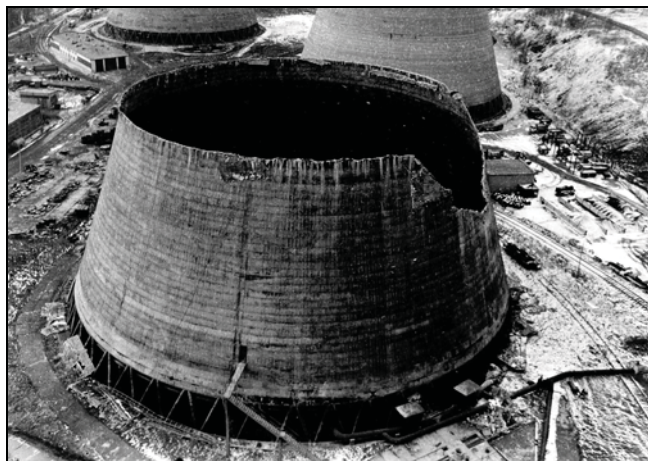
Fig. 1 RC Cooling tower after the collapse
