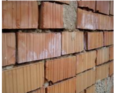
Figure 6. Efflorescence in the brickwork
