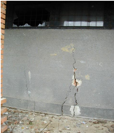
Figure 1. Cracking in the brickwork
