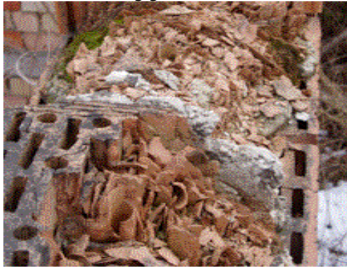
Figure 5. Brickwork of perforated bricks showing frost damage
