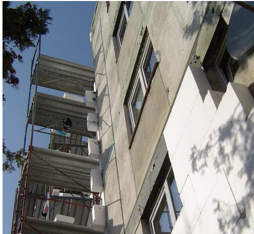
Figure 5. Building from Cluj- Napoca town in the process of rehabilitation with 15 cm of polystyrene EPS
