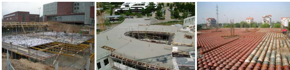
Figure 16. Aspects during casting in place of the concrete slab with spherical gaps
