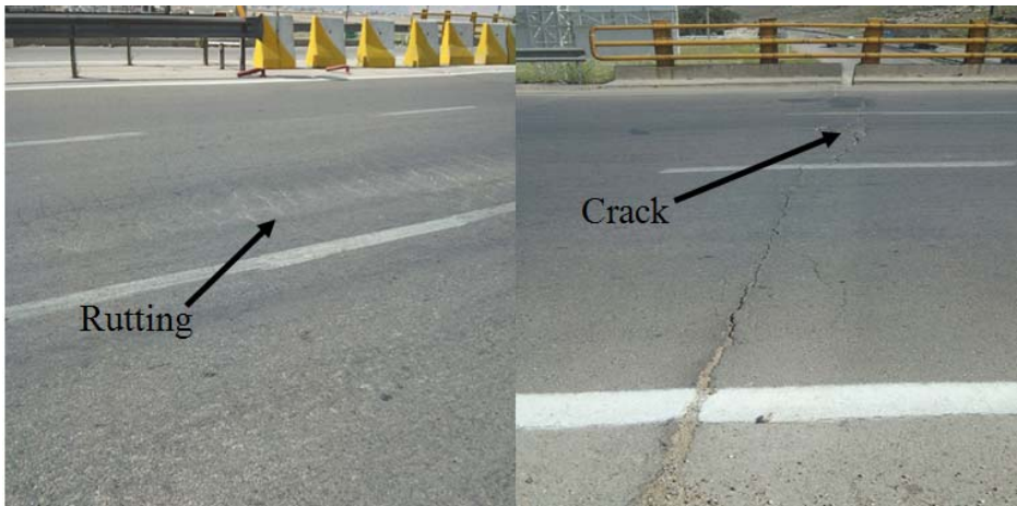
Figure1. Pavement distress on bridge situation (Fasa Bridge)
